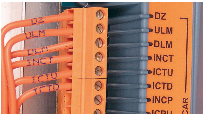
Typical label stamping at controller end
